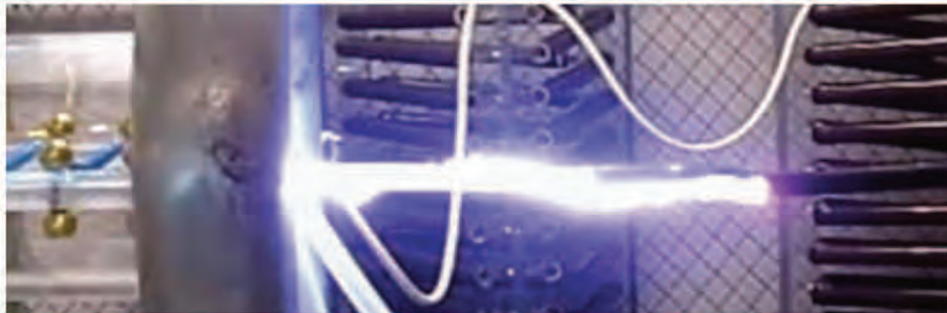
Figure 10. CUT#5. Photo of flashover. Positive polarity.
